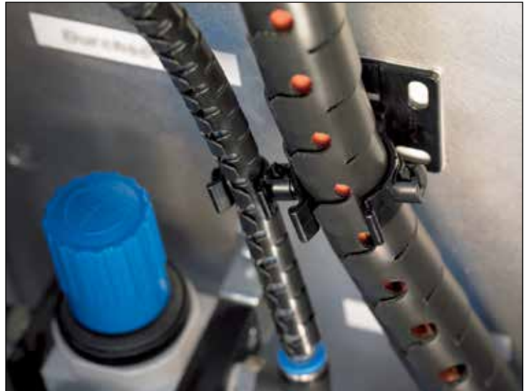
For example: The protection and affixing of cables in a wiring cabinet with Helawrap sleeving.
